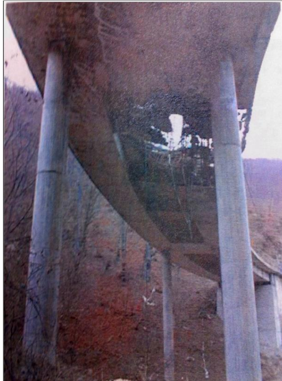
Figure 3-1: Deck and box girder damage on the Kumar II bridge (Honorio, Wight, Erki, & Heffernan, 2003)
