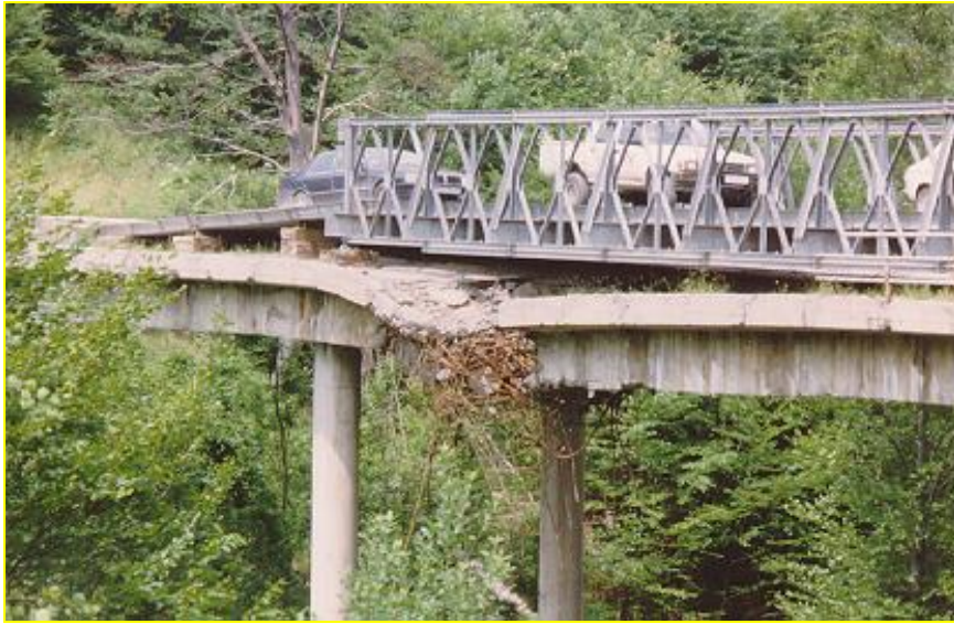
Figure 1-1: War damaged and temporarily repaired bridge in Komar, Bosnia (Maj Stevens. MWF)
