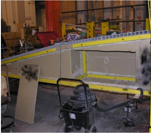
Figure 4-17: Damage Stage 1 (South Side)
