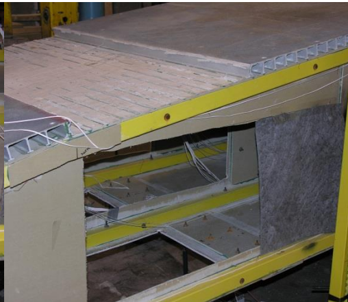
Figure 4-20: Damage Stage 7 West Side
