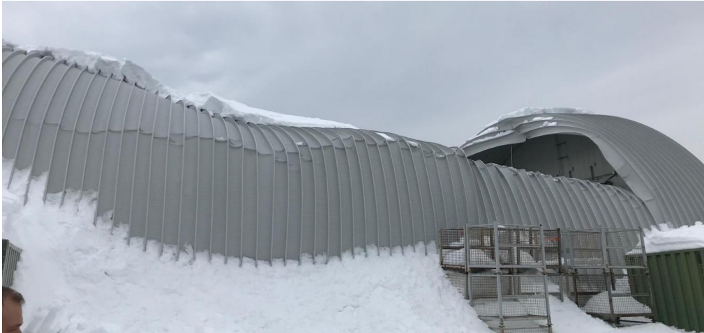
Figure 2-10: Collapse of K-Span in CFB Petawawa
