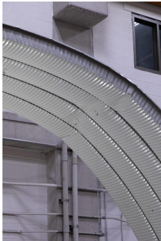
Figure C-42: Unbalanced Loading & Fixed Support Specimen Localized Web Deformations 2
