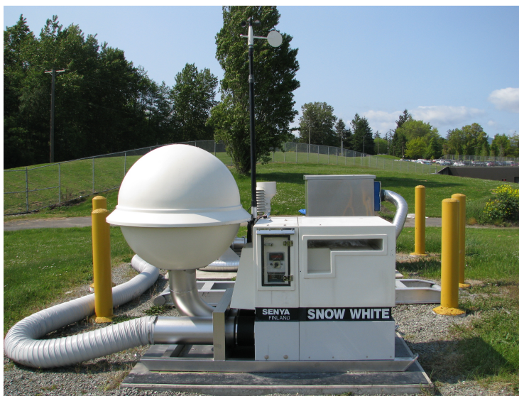
Figure 5.1 – A photograph of the manual CTBT monitoring site (CAP14) in Sidney, Canada. Aerosols enter the sampler through the long tube, drawn in by a pump in the main body. The main body contains state-of-health monitoring equipment and controls the pumping rate to ensure constant airflow. The filter is located inside the dome and the air leaves the air sampler through the flange at the midpoint of the dome.
