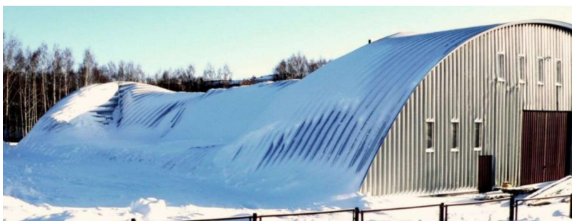
Figure 2.29 - Collapsed K-Span structure in Russia [13]
