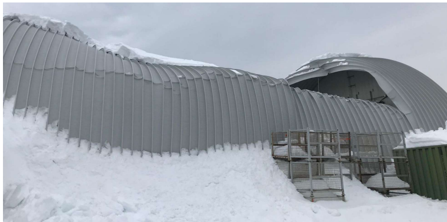
Figure 1.2 - Collapsed K-Span structure in CFB Petawawa [3]
