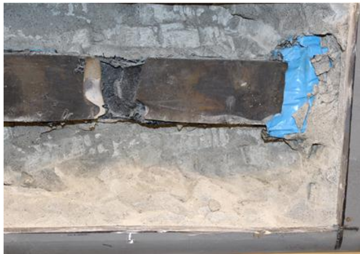
Figure 3.33 –Yield section taper bearing face grout failure
