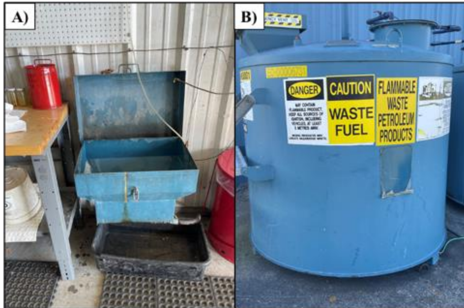
Figure 6.6: Overview of Waste Fuel Storage System A) Waste fuel collector, and B) Waste Fuel Storage Tank
