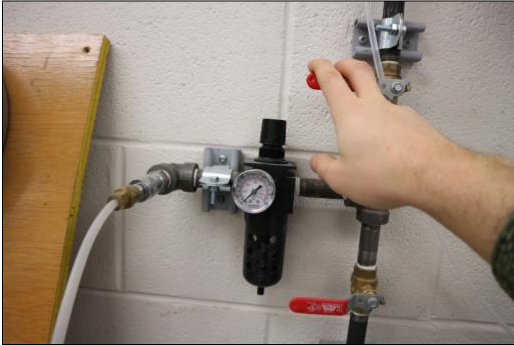
Figure D-88: Turning on compressed air supply.
