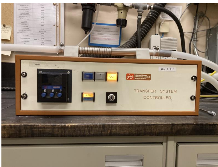
Figure H-1. Sample Transfer System Controller
